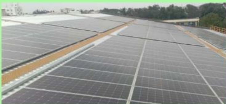
Thamarai Spinning Mills - 100 KW
